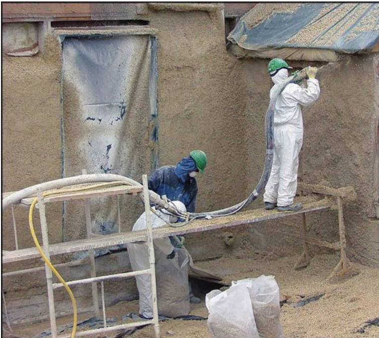
FIGURE 7.32 Spray application of hemp–lime composite to a building. Photo courtesy of Steve Alin.
